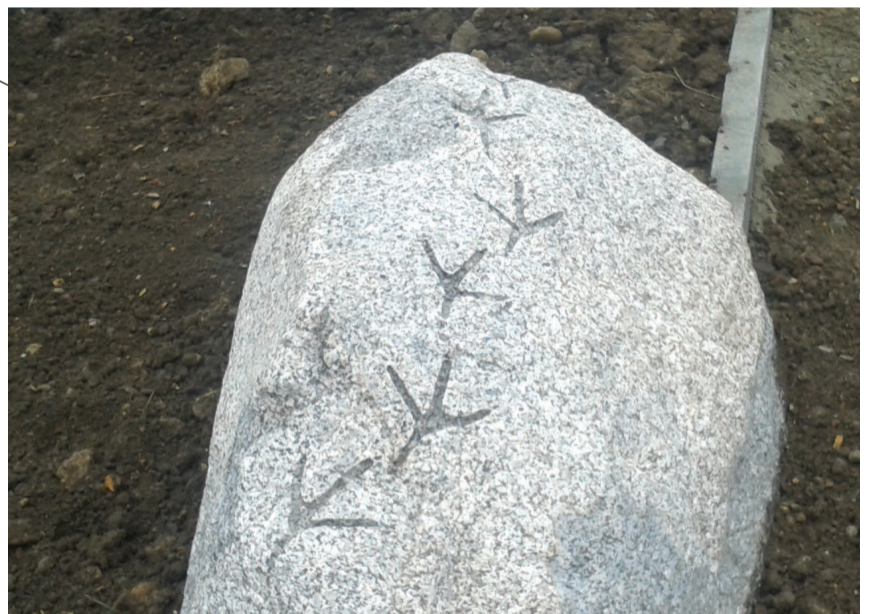
Boulders installed between trees and footpath to form a 'play on the way' track for children and to stop vehicles from entering the site. Subtle patterns on the boulders link to wildlife on the New River.
